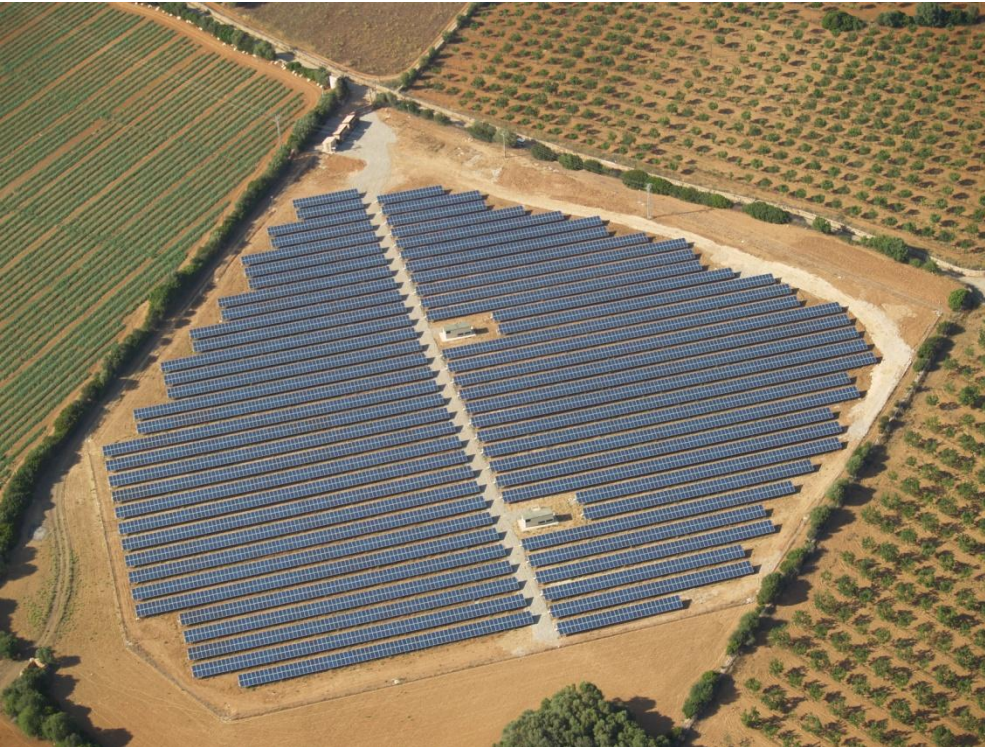
Cortadeta (ES) 2'214.8 kWp
